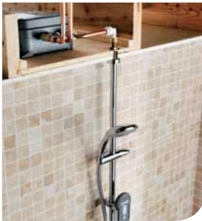
Loft installation - convenient for water inputs and ceiling connection to shower
